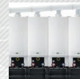
Condensing Cascade Boiler
